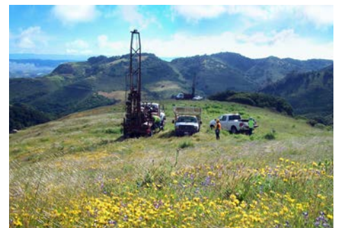
Lompoc Wind Energy Project
