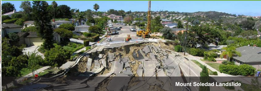
Mystic Lane Landslide
