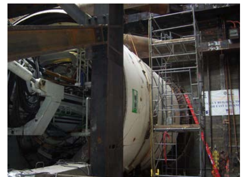
Los Angeles County Metropolitan Transportation Authority Gold Line
